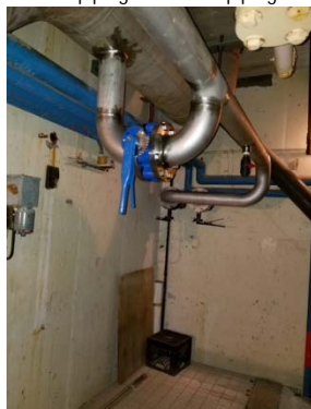
Aeration piping – 4" to 14" piping/valve
