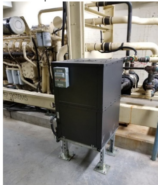
Block Pump Generator Block Heater
