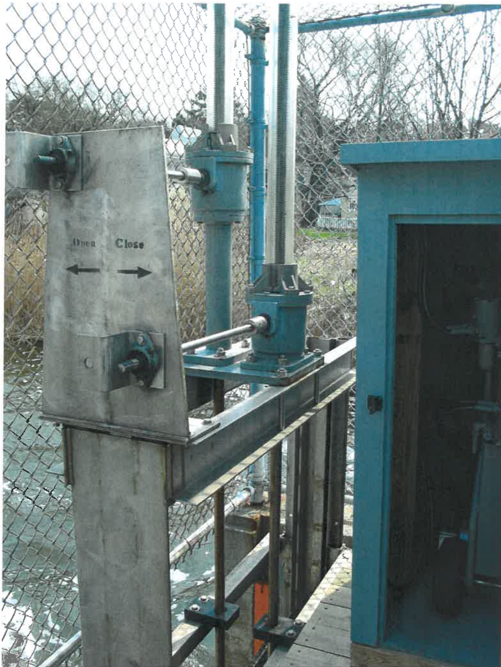
Photo 3. Gate control mechanism.
