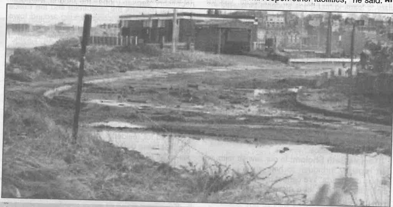
Street flooding due to dune overtopping caused by low dune volume at Phipps Street. [Courtesy photo]
