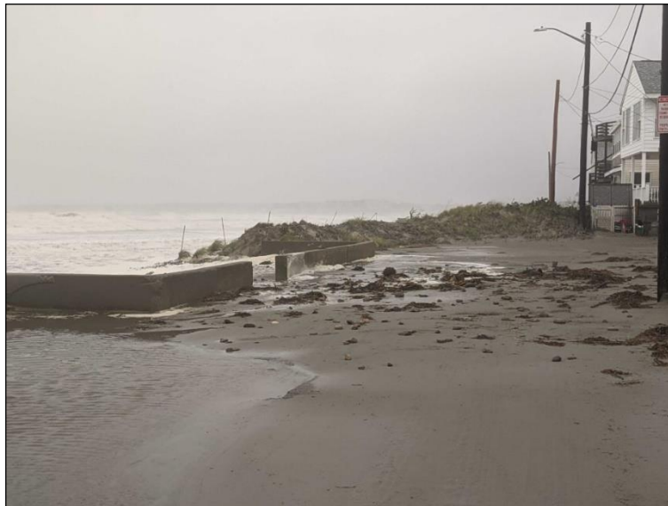
Figure B-9. Photograph following the October 27 th , 2021 Nor'easter showing overwash and sand deposition in the roadway adjacent to the dune gap (patio) at 31 Beach Ave.
