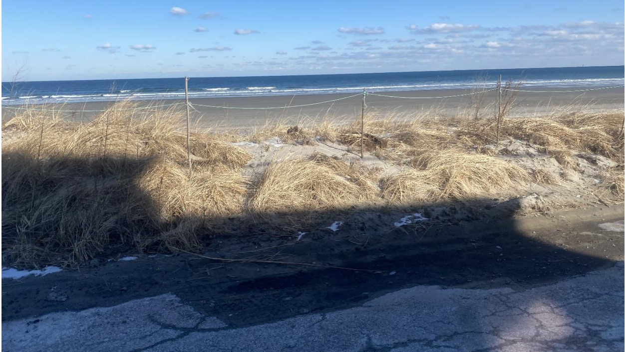
Figure B-14. View of degraded primary dune extending between the gaps adjacent to 33 Malta Street and 31 Beach Ave.
