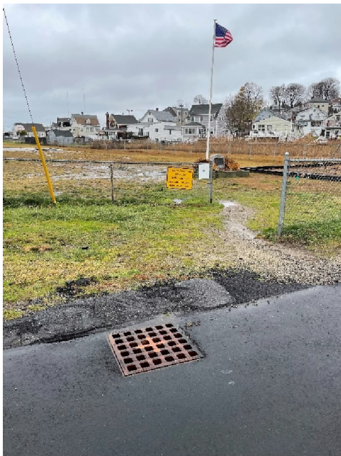
Photo C – Wash out observed to right of CB-1750 where road runoff enters the site
