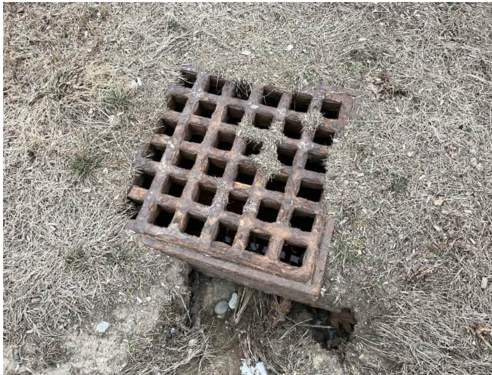
View of catch basin west of the swing set with significant erosion.
