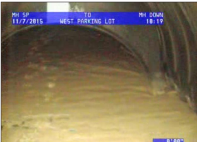
SEPARATOR ROW: Separator Row prior to cleaning
