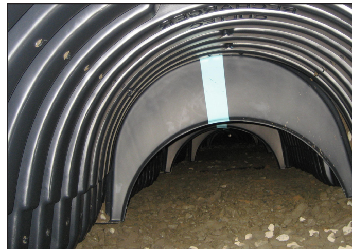
ADJACENT ROW: When the Separator Row is working properly, the adjacent rows will not show signs of sediment.
